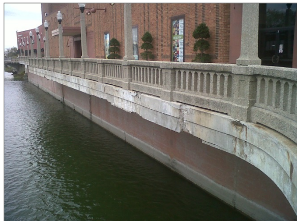
Spalls on Fascia of Edge Beam
