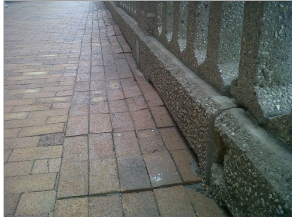
Uneven Brick Pavers at Paramount
