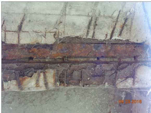
Steel Deterioration at Expansion Joint
