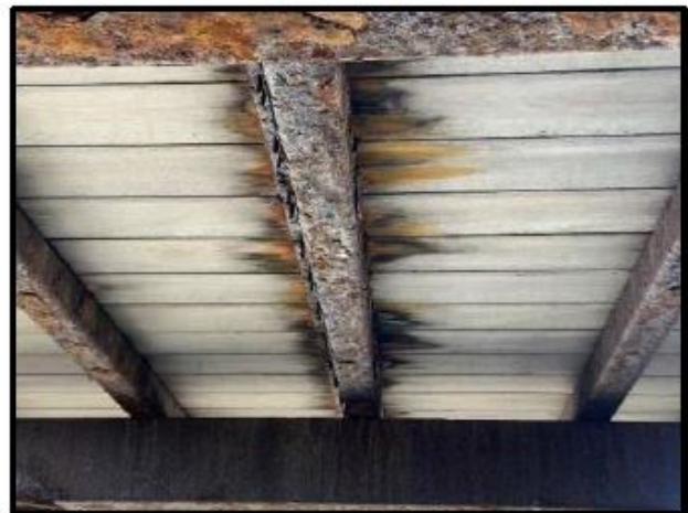
Pack Rust and Section Loss in Stringer
