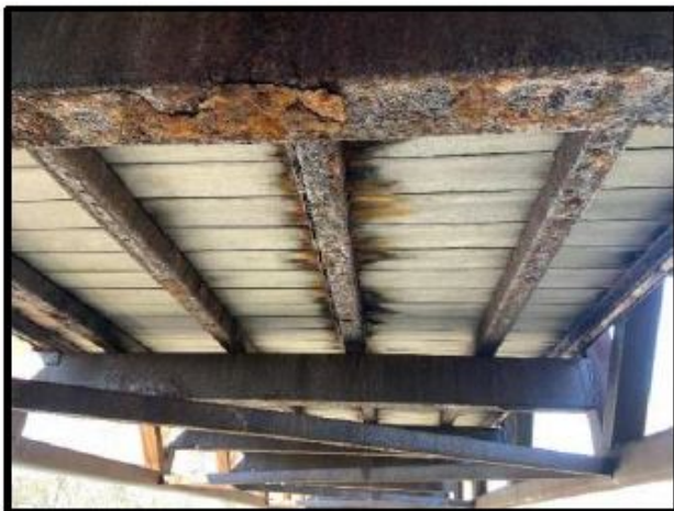
Typical Steel Deterioration
