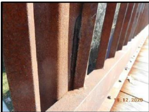
Pack Rust at Weld Between Picket and Tube
