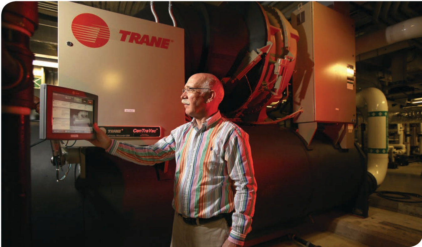
Optimized for energy efficiency, a centrifugal chiller replaced the Butterworth absorption chiller.
