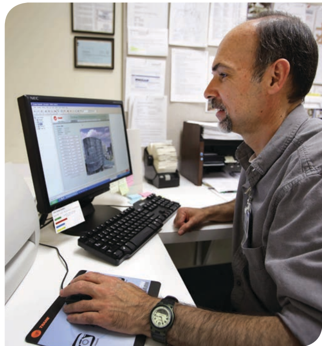
A Trane Tracer Summit building automation system provides an integrated graphical interface with HVAC equipment.
