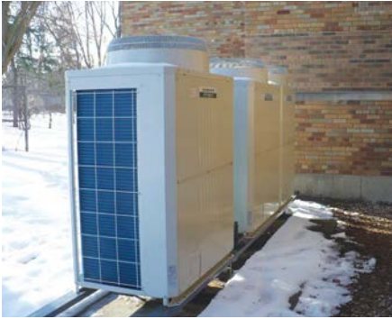
An ultra-high efficiency heating and cooling system is installed at the school district administration center.
