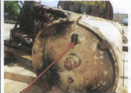
Balance tube fitting. Closer view of missing balance tube.
