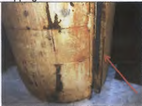
Missing section of balance tube. Balance tube steel channel also missing in same area.
