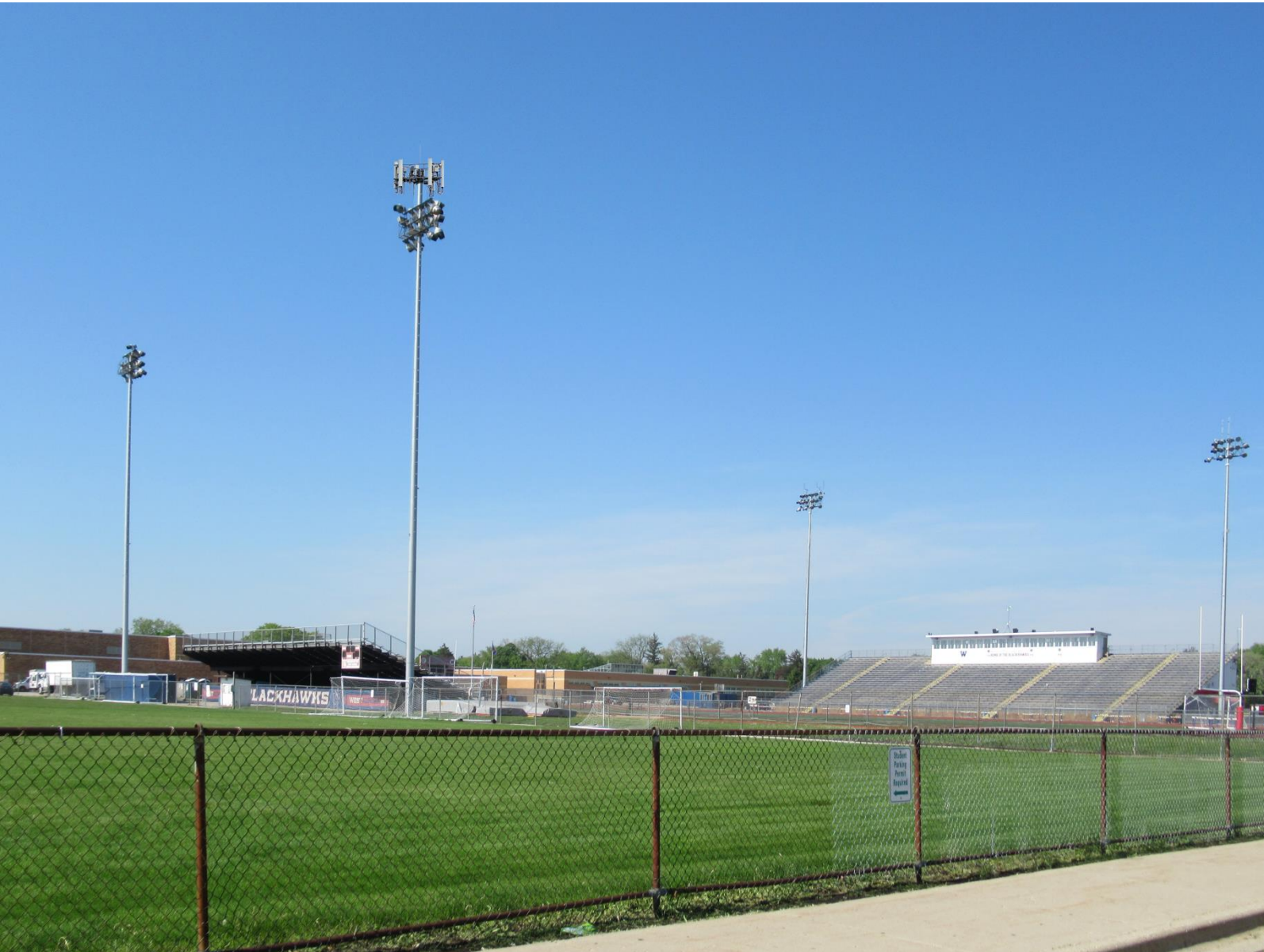
Northeast View (looking Southwest) of T-Mobile Installation on Replacement Stadium Light Pole
