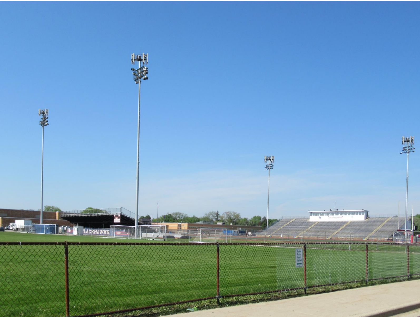
Northeast View (looking Southwest) of (4) Replacement Stadium Light Poles with Carrier Antennas
