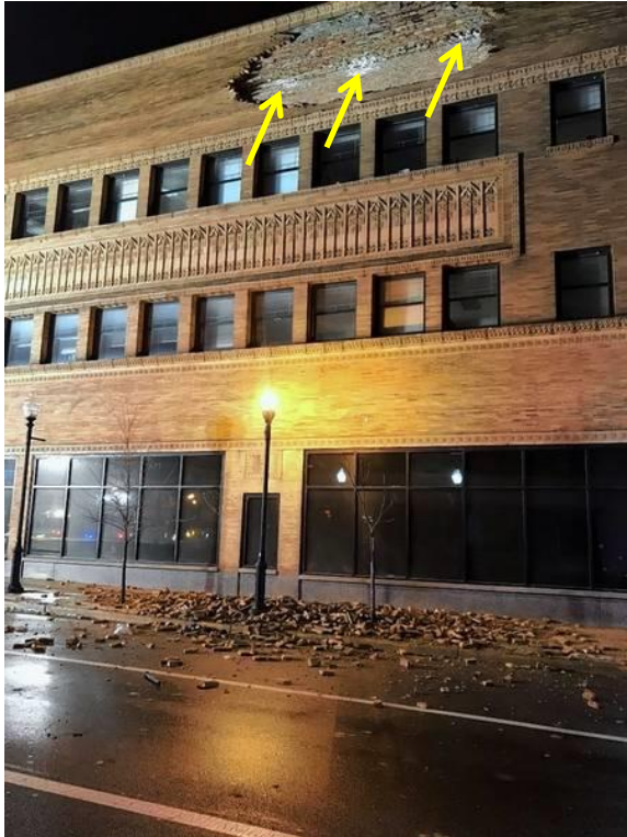
Figure 5. Conditions on February 20, 2019 shortly after brick fell; note what appear to be efflorescence or frost spots on backup masonry (arrows) (photo courtesy of Aurora Police Department as published in the Daily Herald: https://www.dailyherald.com/news/20190220/galena-boulevard-in-aurora-closed-after-partial-building-collapse )
