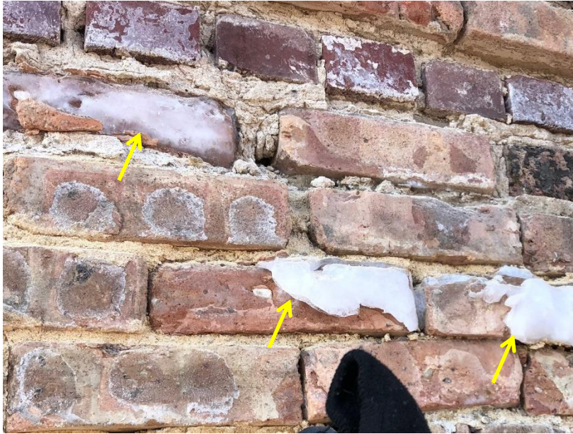
Figure 13. Ice visible on backup brick (photo courtesy of FHP)
