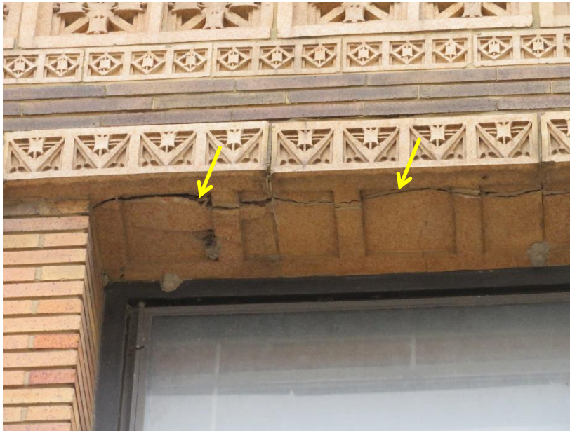
Figure 31. Cracked and spalled lintel units above the second floor windows on the north facade (condition typical at majority of second floor window lintel units on north facade)
