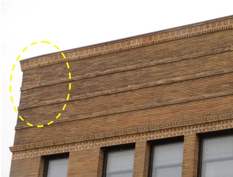
Figure 25. Potential area of bulged face brick at parapet on north facade near northeast corner
