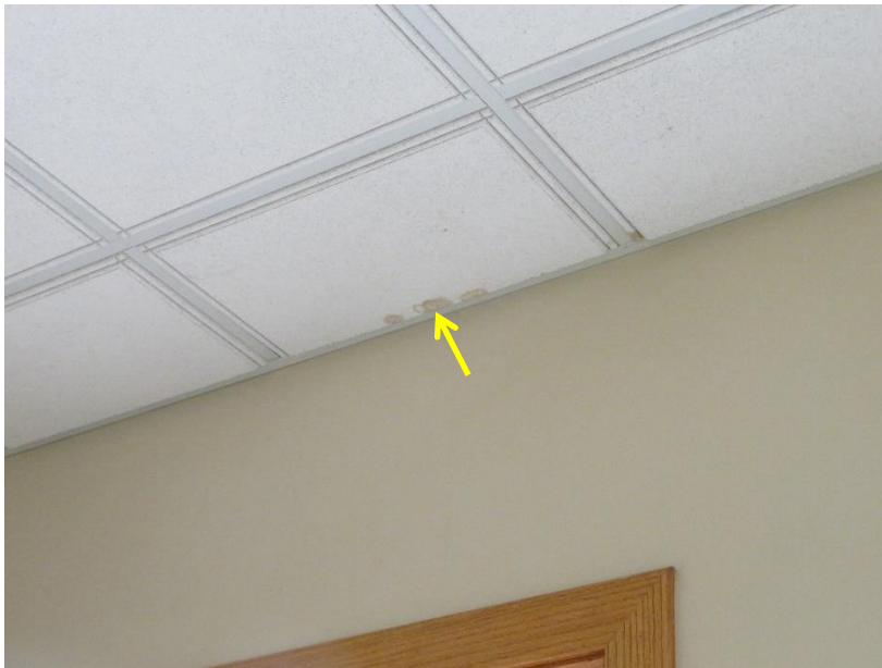
Figure 24. Isolated water marks on the ceiling in third floor space adjacent to the north facade
