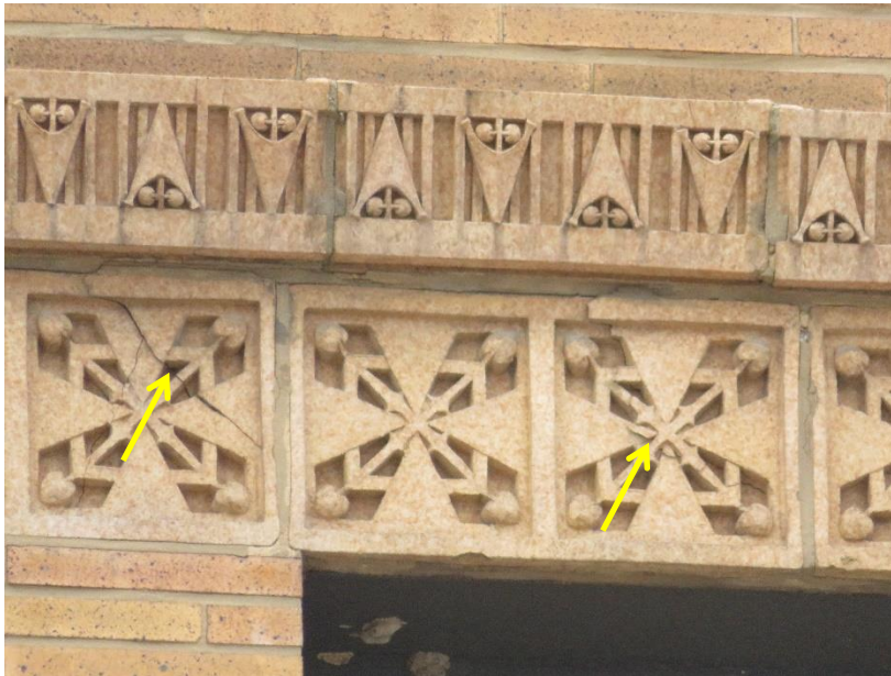
Figure 27. Cracked terra cotta units on east facade above third floor windows
