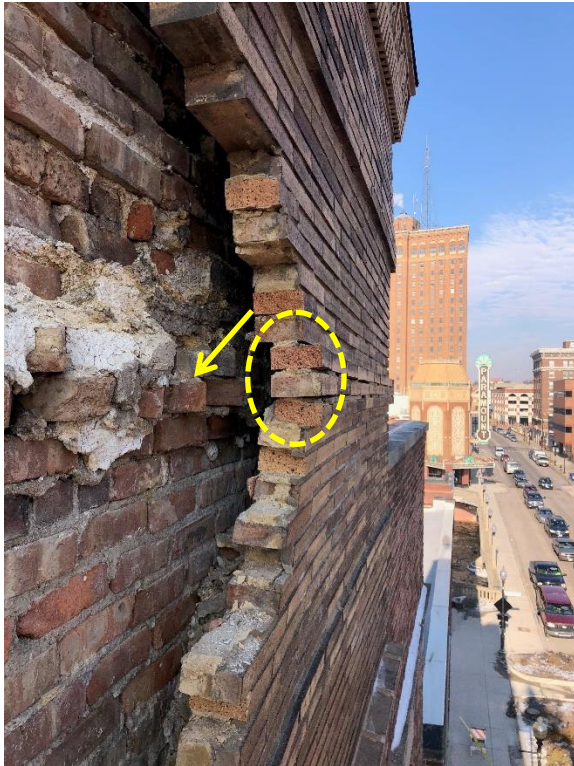
Figure 11. Bulged face brick; backup brick laid diagonally (arrow) corresponds roughly with roof line; the diagonal bricks may have served as blind headers to engage the adjacent projecting courses of face brick (circled) (photo courtesy of FHP)
