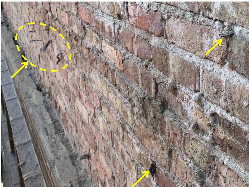
Figure 16. Irregularly spaced and corroded veneer ties below roof line (photo courtesy of FHP)
