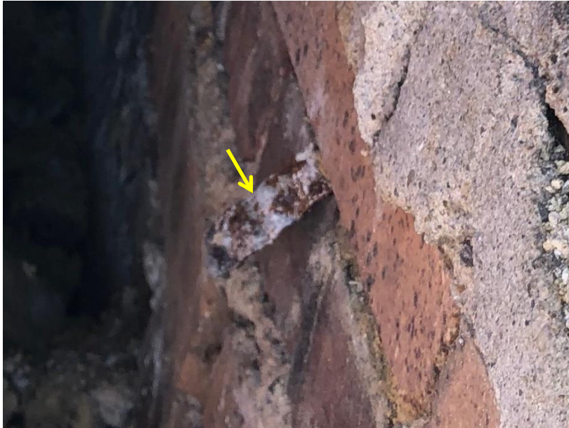
Figure 17. Close-up view of veneer tie with relatively minor corrosion but no engagement with face brick (photo courtesy of FHP)
