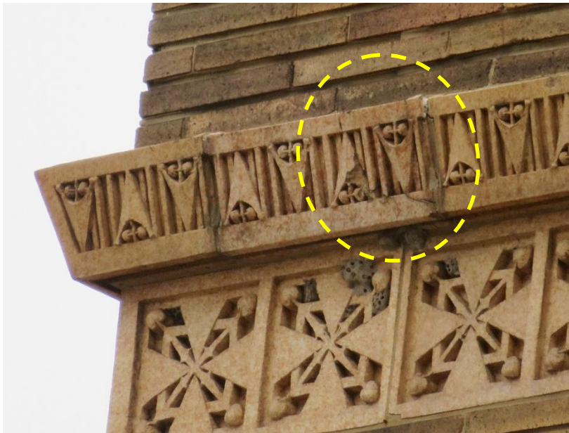
Figure 28. Cracked terra cotta unit on the north facade at the top course above the third floor windows
