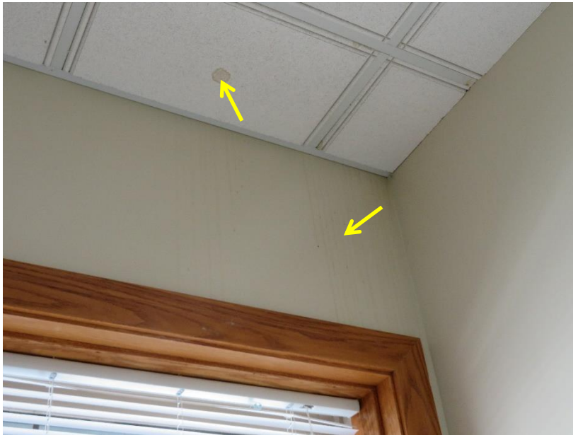
Figure 23. Isolated water marks on the ceiling and wall in third floor space adjacent to the north facade
