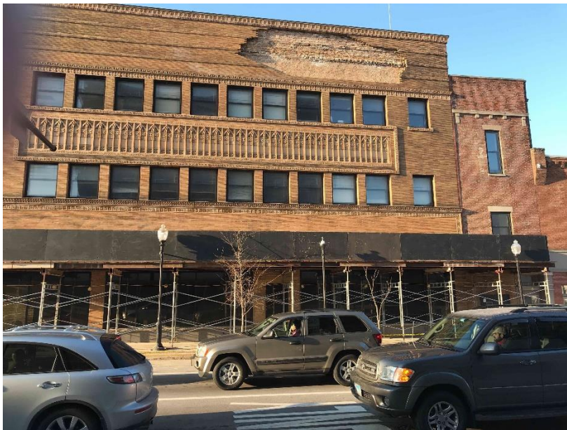
Figure 6. Conditions on February 22, 2019 after removal of additional brick masonry and erection of sidewalk canopy (photo courtesy of FHP)
