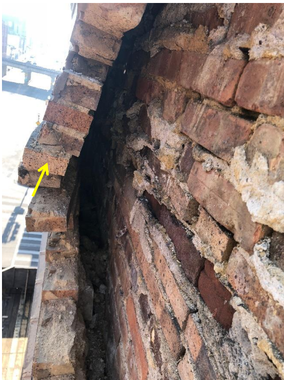
Figure 12. Bulged face brick (photo courtesy of FHP)
