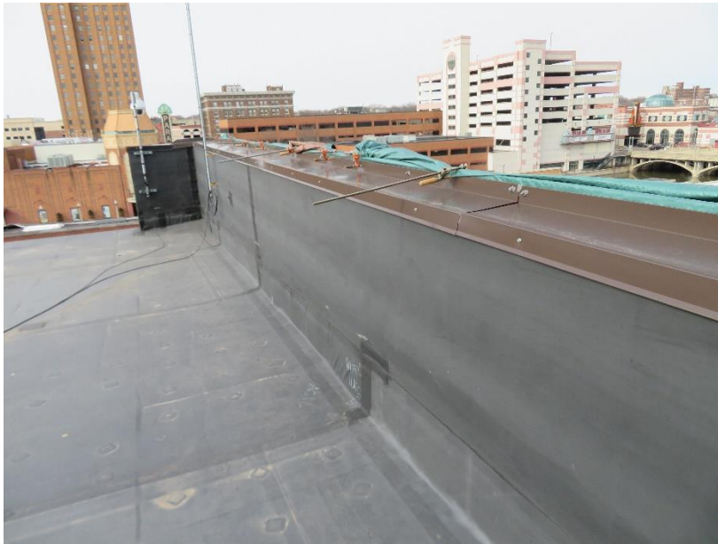
Figure 22. Roof side of the parapet at the area of loss
