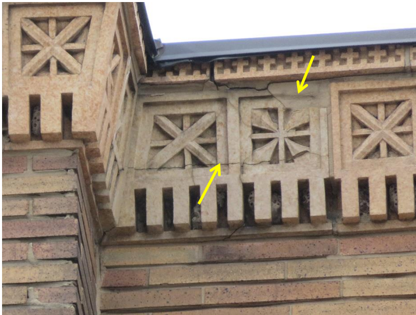
Figure 26. Cracked and previously patched terra cotta unit at parapet on east facade
