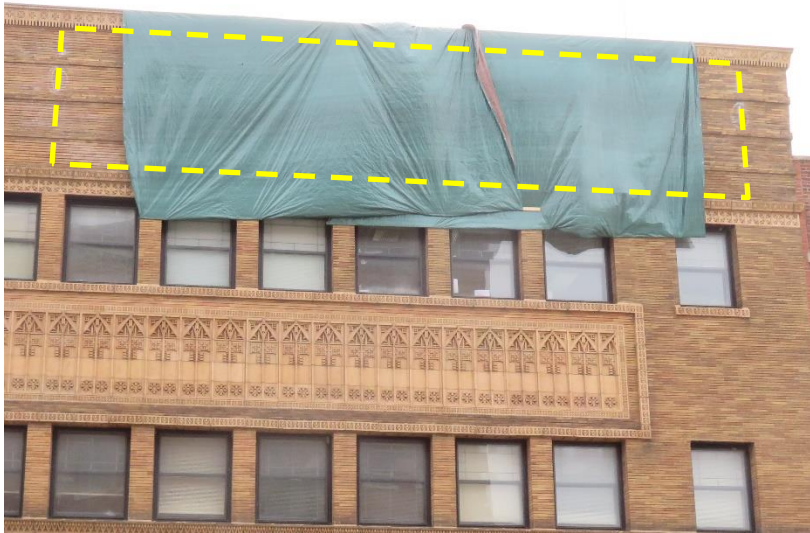
Figure 9. Extents of bulged face brick marked with white chalk by FHP (outline added for clarity)
