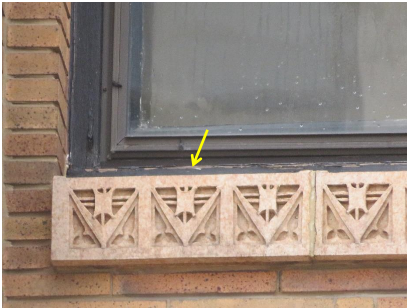
Figure 32. Peeling paint at wood window frame outside of metal storm window
