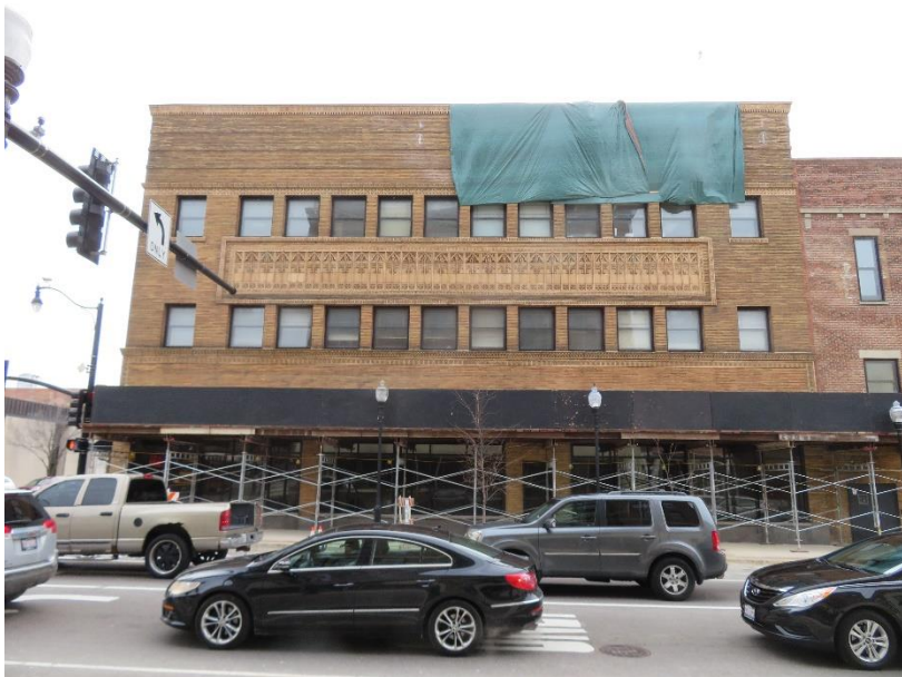
Figure 8. North facade on February 25, 2019; area of loss covered with tarp
