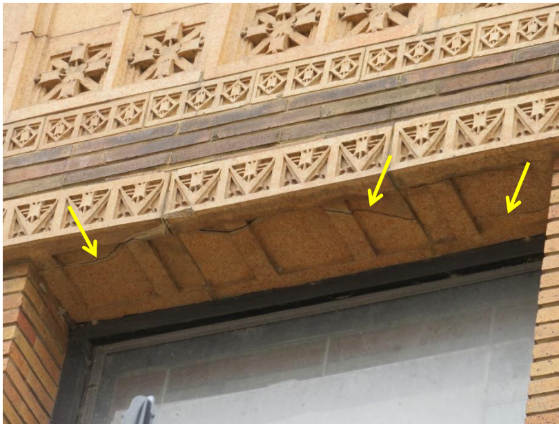
Figure 30. Cracked lintel units above the second floor windows on the north facade (condition typical at majority of second floor window lintel units on north facade)
