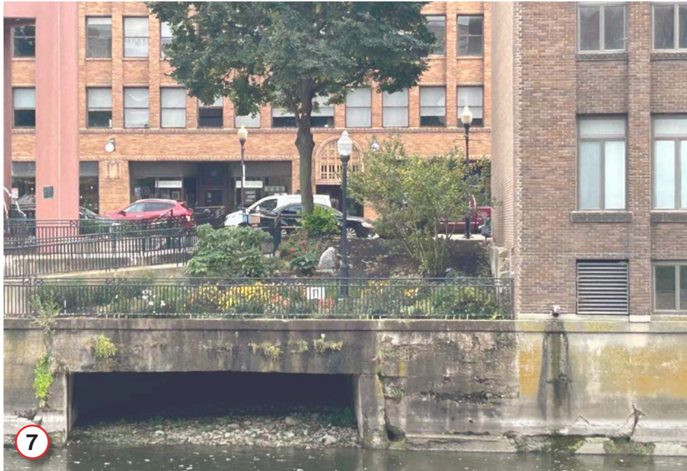
7 There is an existing culvert in the river retaining wall that is a relic of an old mill on site - opportunity to tell this story.
