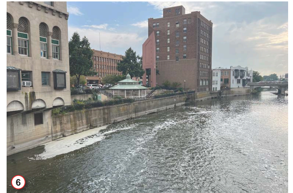
The existing river wall looks to be in poor condition, but a recent structural evaluation confirmed that it is structurally sound.
