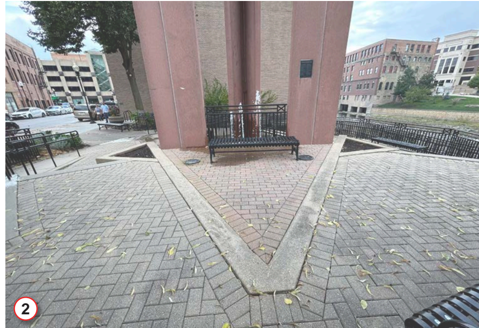
Existing fountain is functional, but is blocked off by guardrails. Existing paver field around monument contains engraved donor pavers. The existing pavers are in fair condition but have faded and lost their color.
