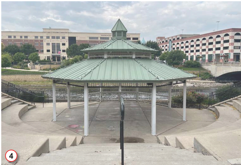
The prefabricated shelter is in fair condition but blocks views of the river.
