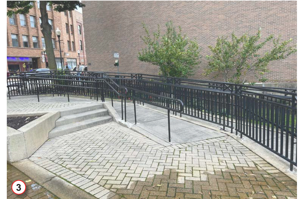
Stairs, ramps, and curbing are in fair/poor condition with visible cracking and chipping. The configuration of the stairs and ramps take up a large area.
