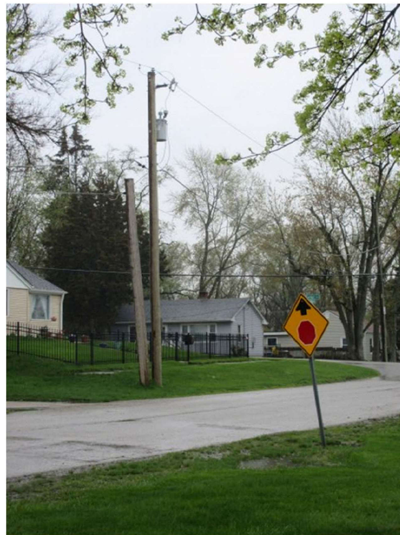
EXISTING UTILITY POLE W/ TRANSFORMER
