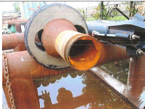
Heavy iron deposition on pipe interior prior to sand blas (typ.)
