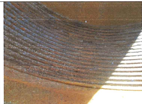
Eroded thread on coupling.
