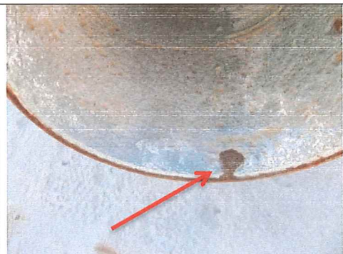
Interior pipe pit above sacrificial zinc anode.
