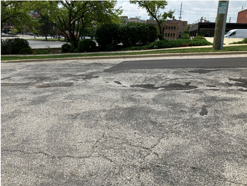
Rough Pavement from Watermain Break (Looking South)
