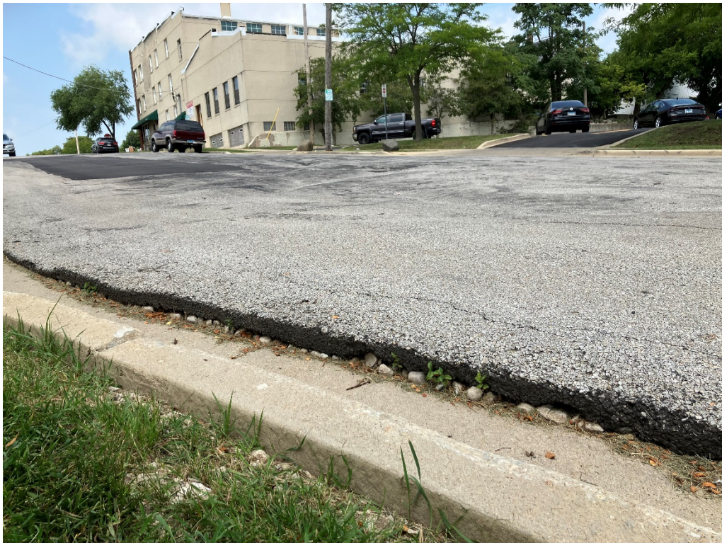
Pavement Heaving around Bank Driveway (Looking North)
