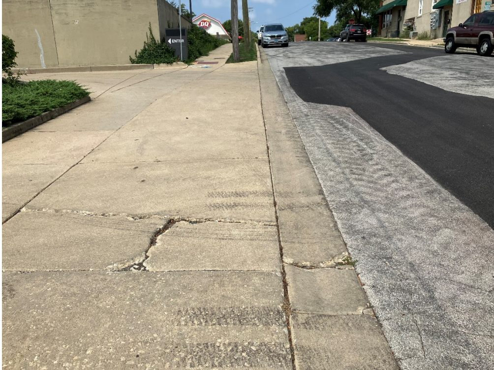
Damage at Bank Driveway (Looking Northwest)
