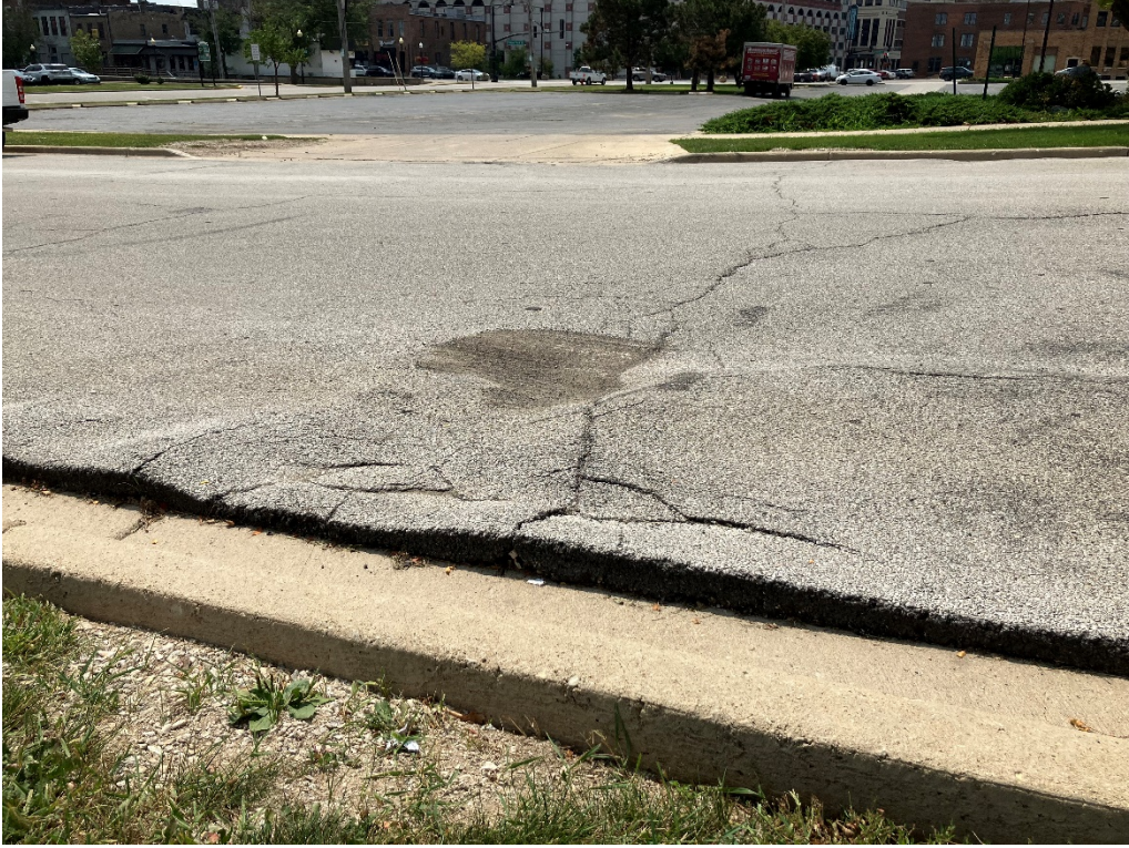
Pavement Heaving (Looking South)
