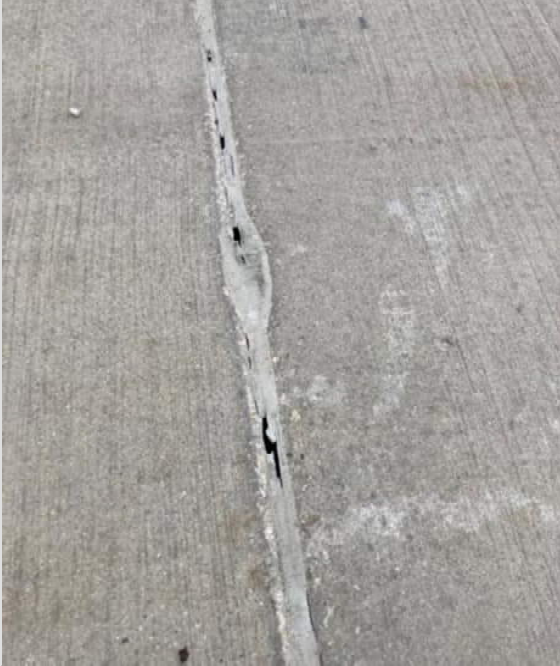
Photo 11 – Widespread failed tee-to-tee joint sealant observed.
