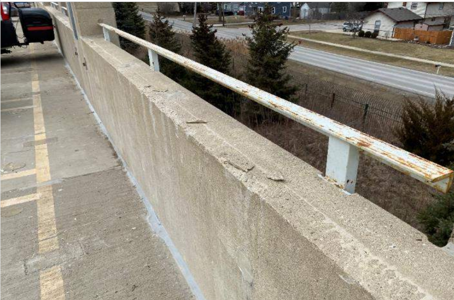
Photo 26 – Metal guardrail attached to top of precast wall along north elevation corroded.
