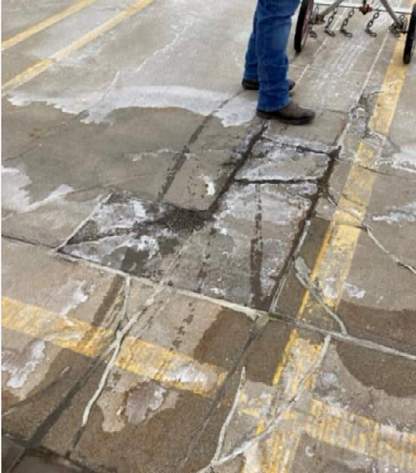
Photo 1 – Typical spalled and delaminated concrete.
