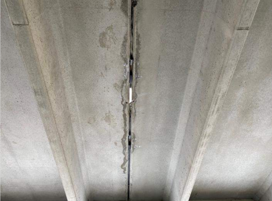
Photo 13 – Widespread failed tee-to-tee joint sealant observed.
