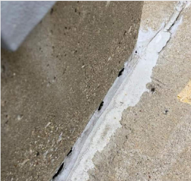
Photo 16 – Adhesion failure to cove joint sealant.
