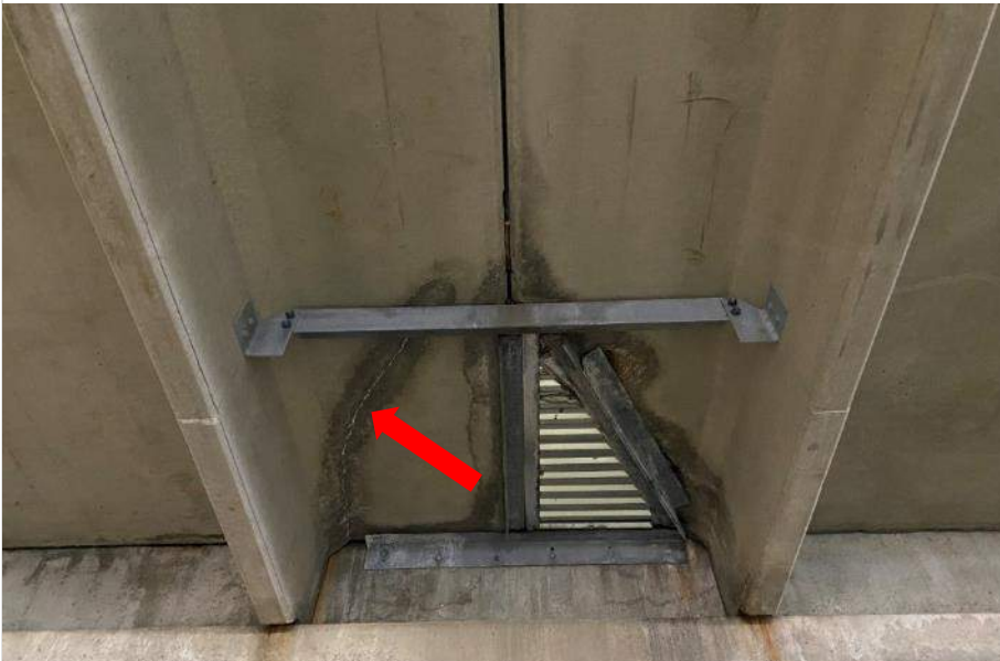
Photo 6 – Full-depth cracking and water infiltration observed at double-tee flanges that were previously repaired.
