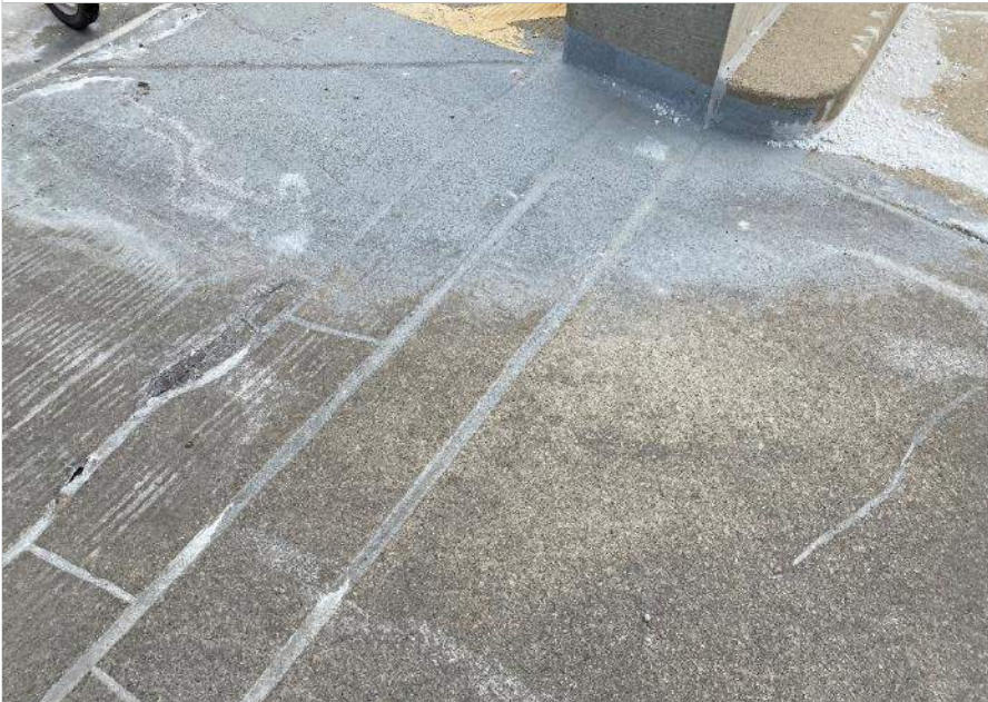
Photo 22 – Traffic bearing membrane on top level worn.
