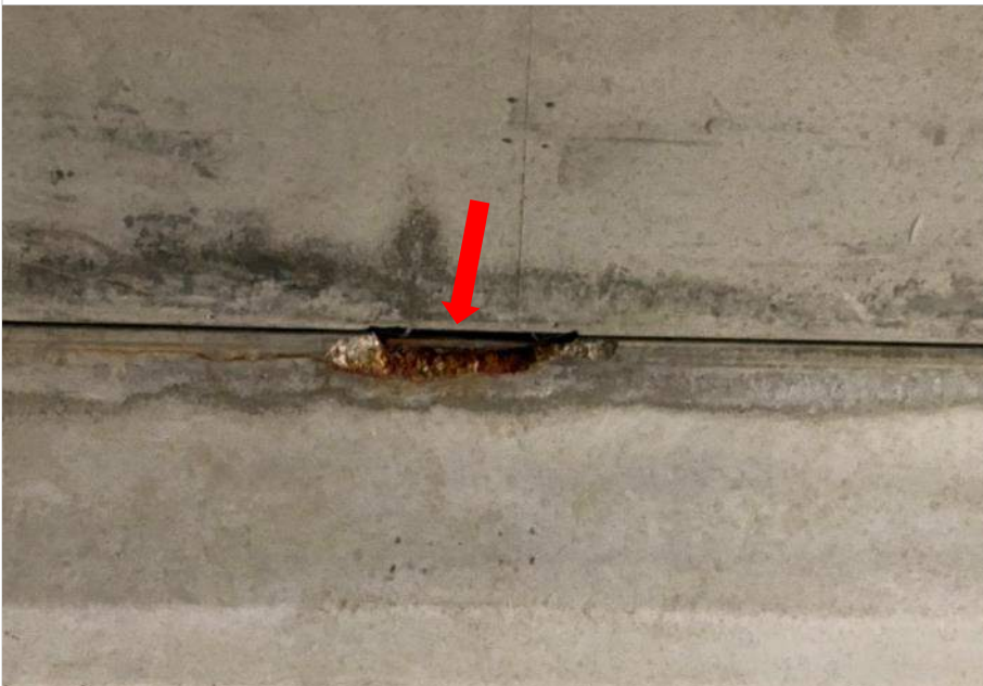
Photo 24 – Corroded double-tee shear connector noted.
