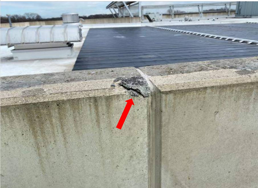
Photo 8 – Isolated spall concrete at precast wall panels observed.
