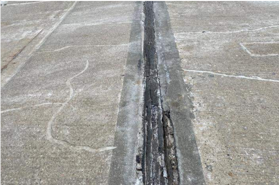
Photo 18 – The parking structure expansion joint has failed. Delamination/spalling in the elastomeric concrete headers was also observed.
