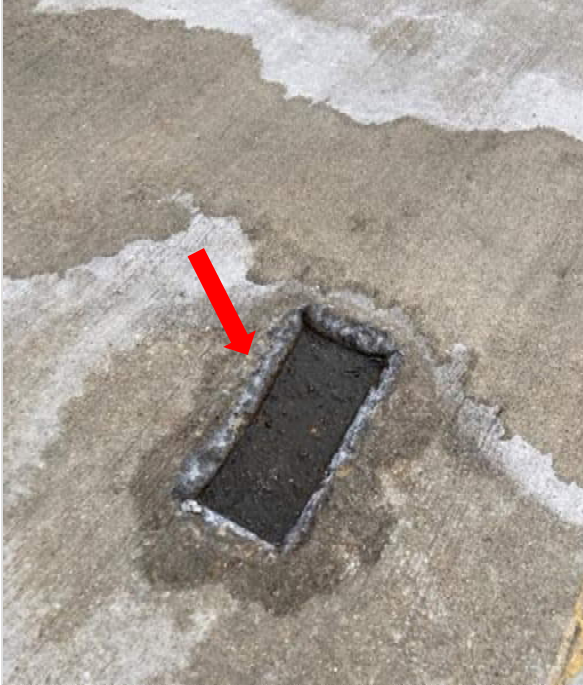
Photo 3 – Typical delaminated concrete at lifting loop pockets.
