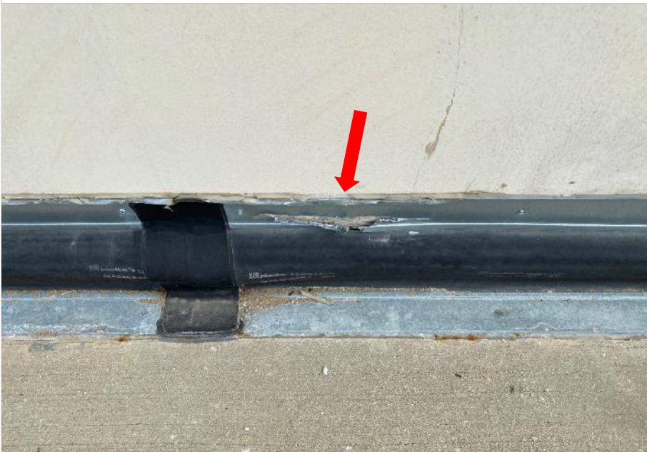
Photo 20 – Sealant at precast wall panel failed.
