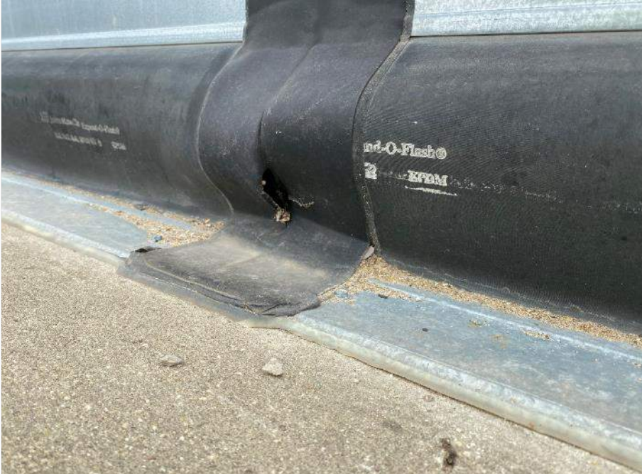
Photo 21 – Joint boot in expansion joint punctured.
