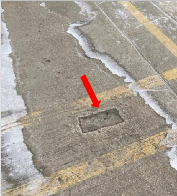
Photo 4 – Deteriorated concrete at a curb on the top level.
