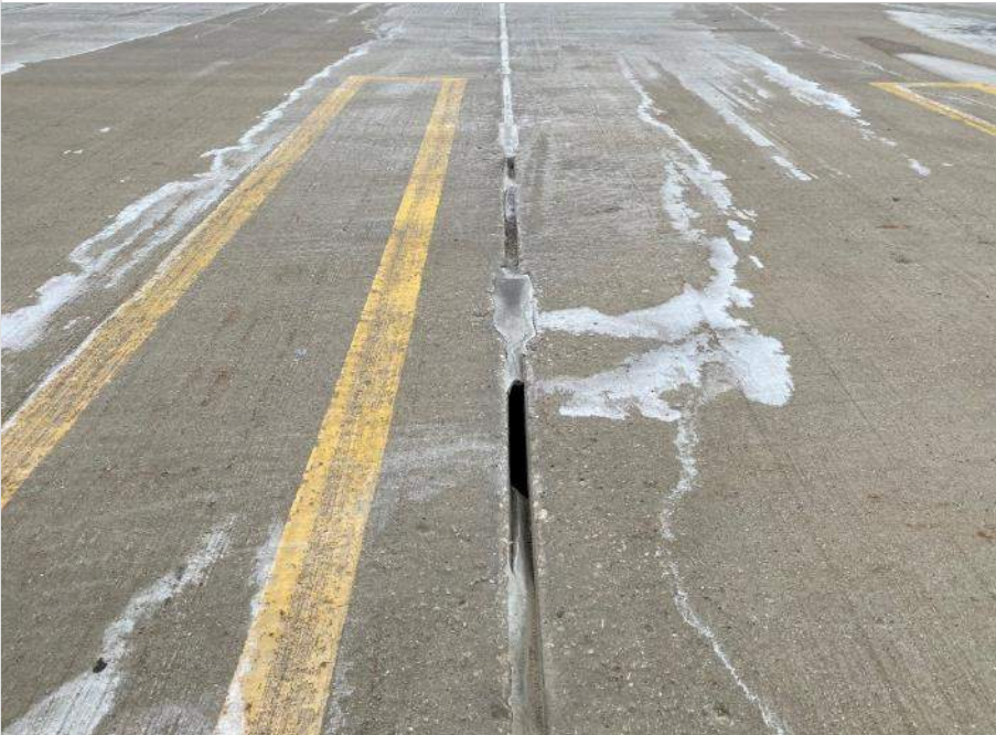
Photo 10 – Widespread failed tee-to-tee joint sealant observed.
