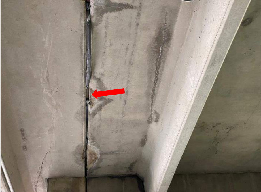
Photo 23 – Broken double-tee shear connector observed (welds broken).
