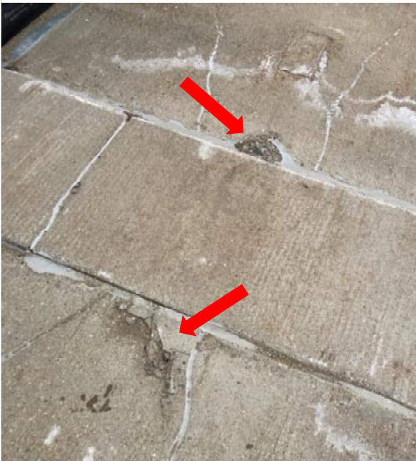
Photo 2 – Typical spalled and delaminated concrete.
