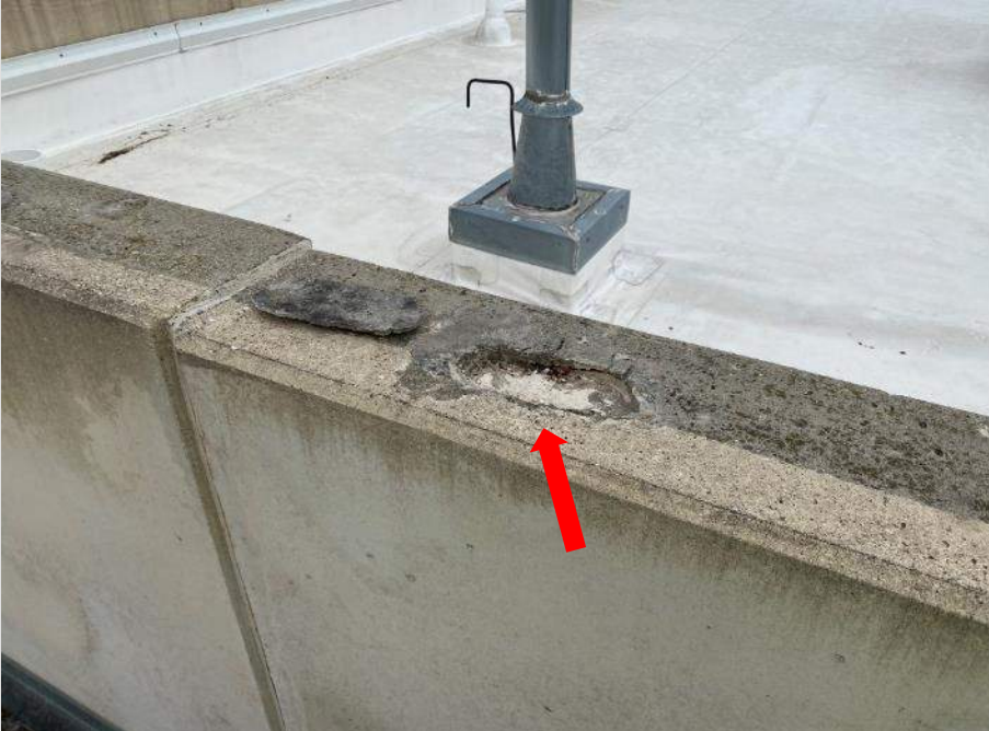
Photo 9 – Typical delaminated concrete observed at a precast wall.
