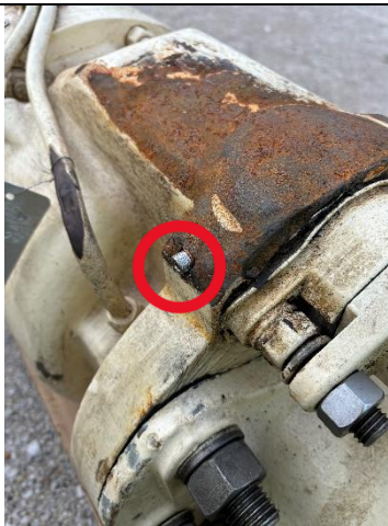
Unguarded vent screw w/ paint rubbed off
