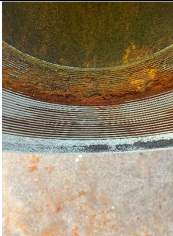
Improper thread engagement depth in coupling
