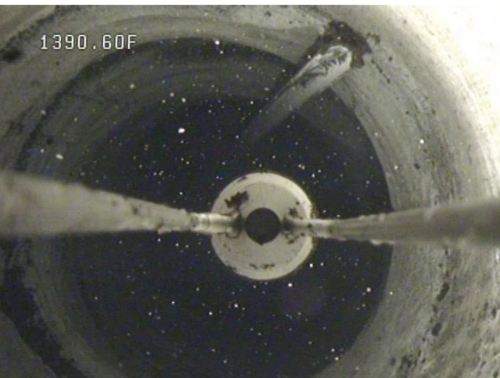
1390' Top of broken PVC at bottom
