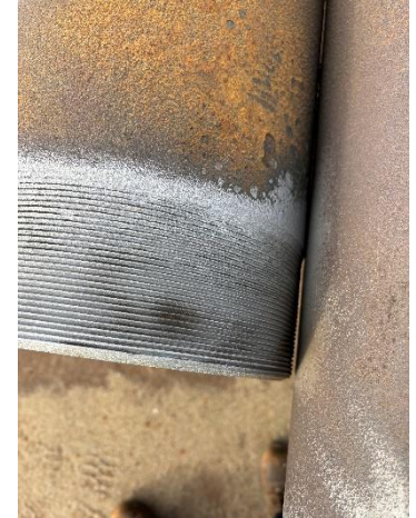
Short thread engagement and thread deterioration
