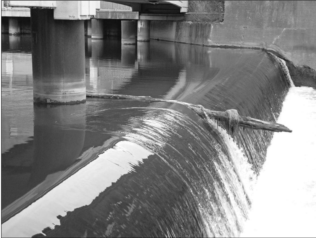
Photograph 17. View of the Timber Debris over the Dam near Station 0+50, Looking East.
