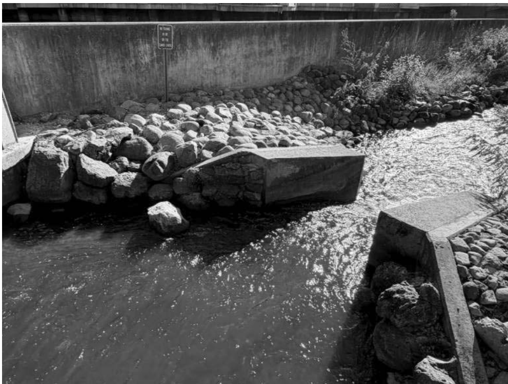
PHOTOGRAPH DS2-2: EROSION AT DS2 UPSTREAM RIPRAP
