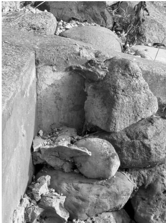
PHOTOGRAPH DS3-2: TYPICAL EROSION CONDITION
