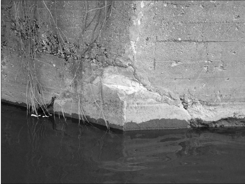
Photograph 19. View of the Scaling at the East Abutment Upstream of the Dam, Looking Southeast.
