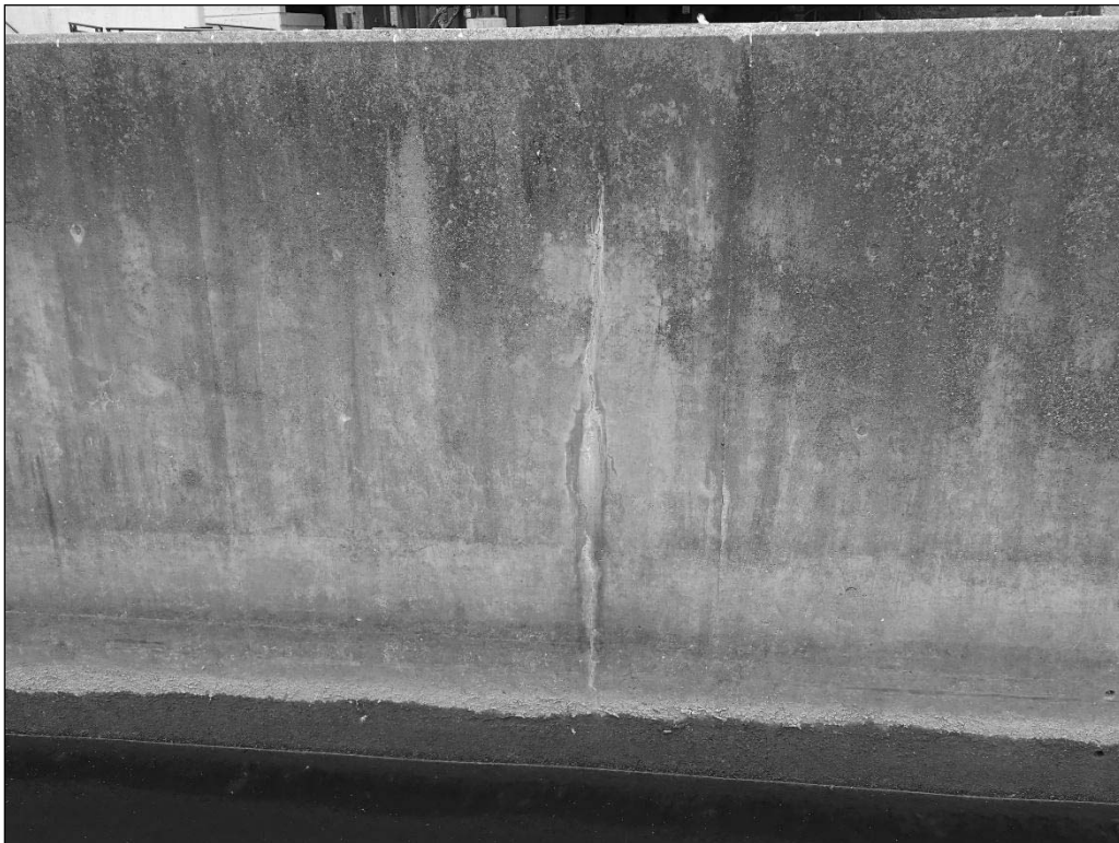
Photograph 16. View of a Typical Crack on the East Face of the Canoe Chute East Wall, Looking West.
