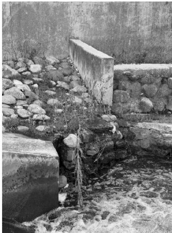
PHOTOGRAPH DS4-4: DS4 DOWNSTREAM EROSION
