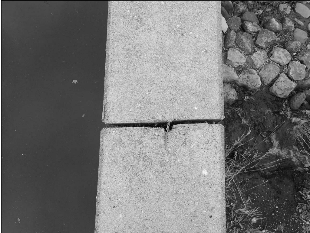
Photograph 13. View of the Top of the Canoe Chute East Wall at Station 1+80, Looking South. Note Active Water Flow on the West Side of the Wall.
