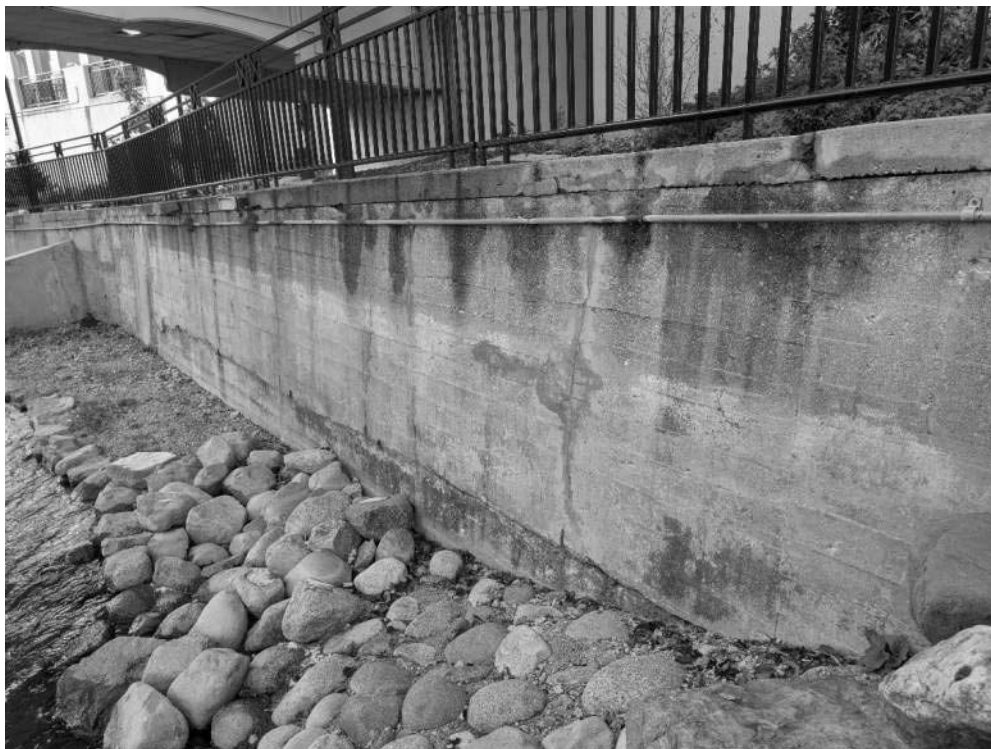
PHOTOGRAPH DS4-6: CRACKING ON DOWNSTREAM CANOE CHUTE WEST WALL
