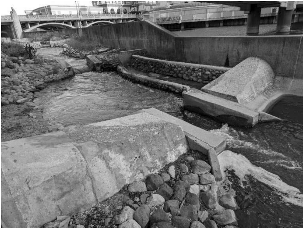
PHOTOGRAPH DS5-2: CRACKING AND SPALLING AT DS5
