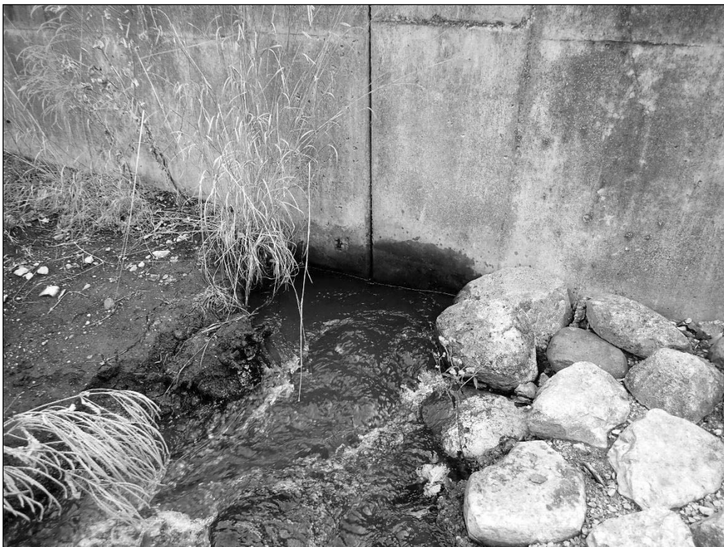
Photograph 14. View of Active Water Flow and Bank Erosion on the West Side of the Canoe Chute East Wall at Station 1+80, Looking East.
