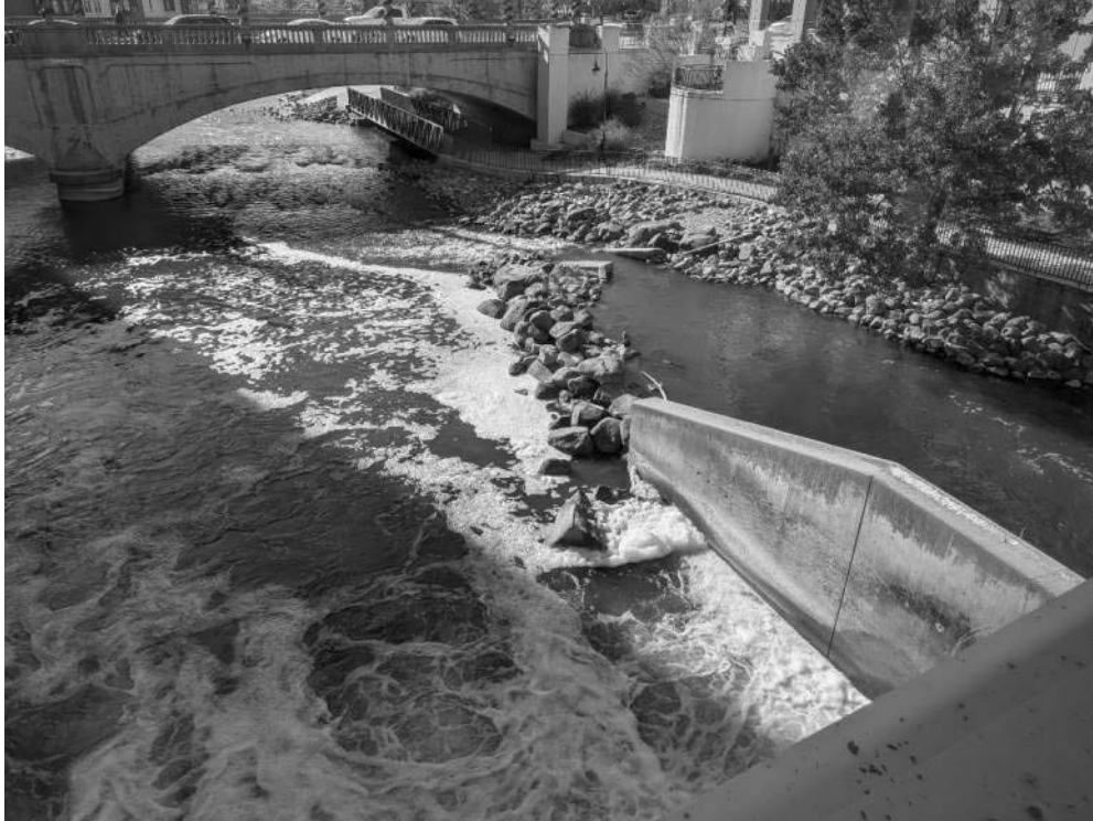
PHOTOGRAPH OUT-3: LOOSE RIPRAP/CONCRETE CANOE CHUTE EAST WALL ON FOX RIVER SIDE
