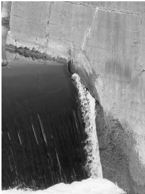
PHOTOGRAPH WD-5: WEST DAM FOX RIVER EAST WALL SCALING DETAIL
