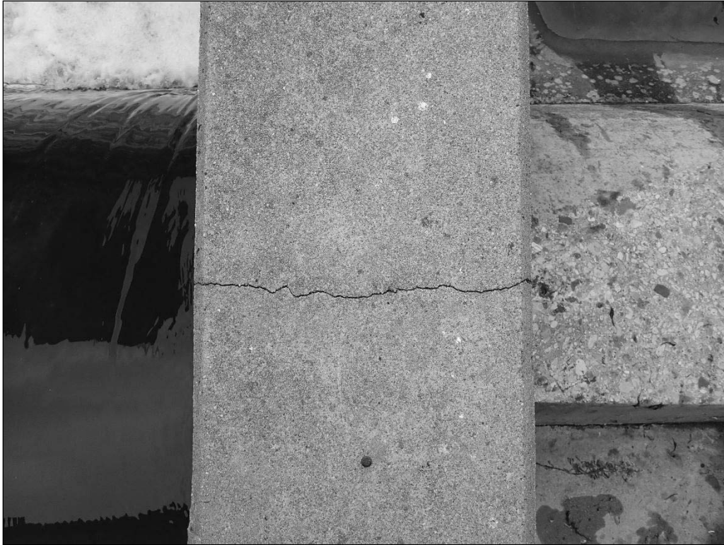
Photograph 15. View of a Typical Crack across the Top of the Canoe Chute East Wall, Looking South.
