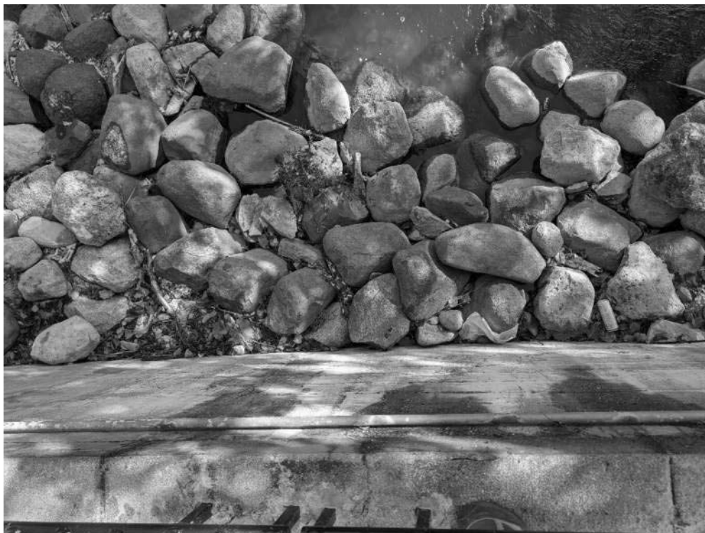
PHOTOGRAPH DS5-4: CRACKING IN CANOE CHUTE WEST WALL
