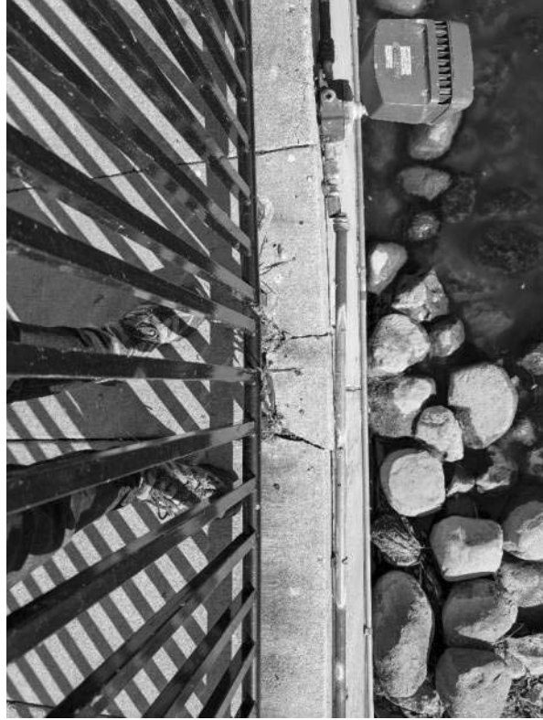
PHOTOGRAPH DS3-3: CRACKING IN SIDEWALK AT CANOE CHUTE WEST WALL
