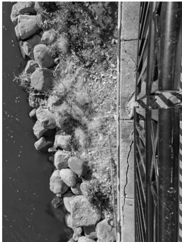
PHOTOGRAPH DS3-4: CRACKING IN SIDEWALK AT CANOE CHUTE WEST WALL
