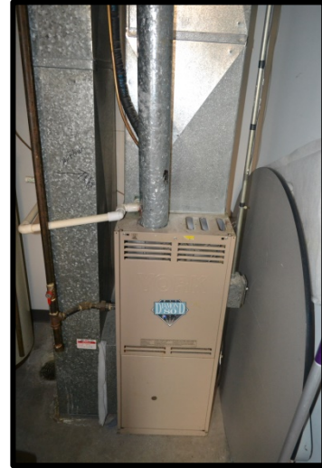
View of a furnace
