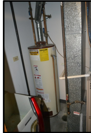
View of the water heater
