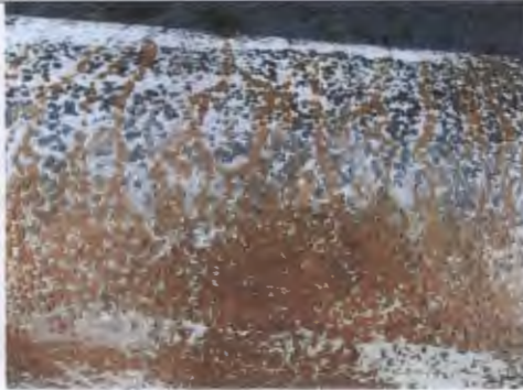
The 10' length has a "rash" of pitting throughout its length...
