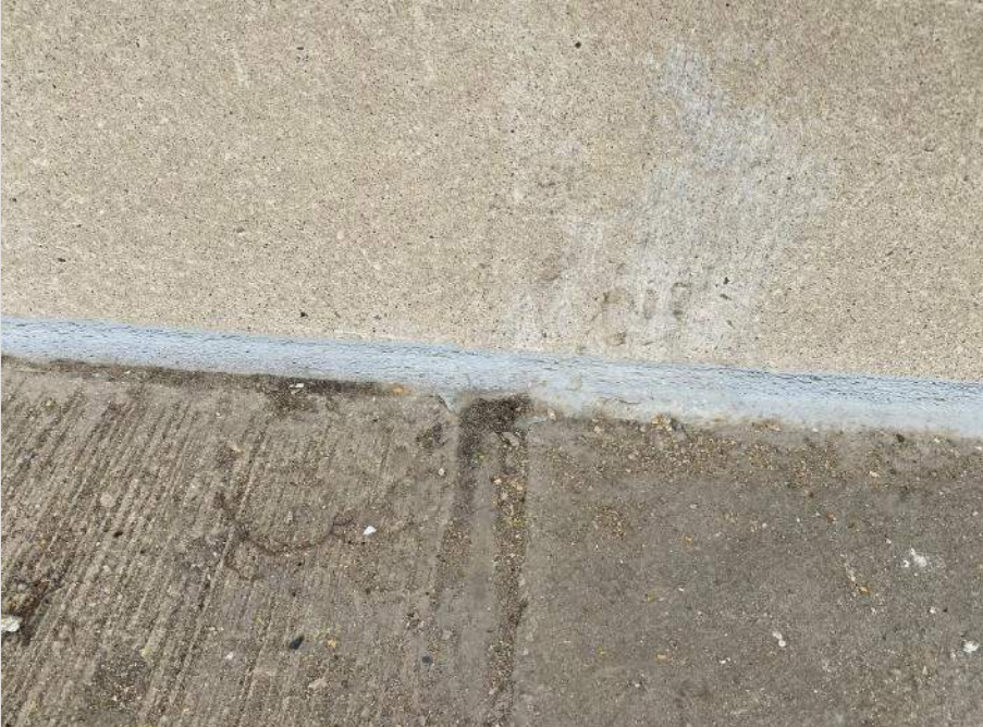
Photo 15 – Drying and shrinkage cracks noted in cove sealant.
