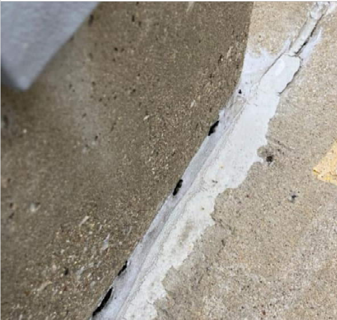
Photo 16 – Adhesion failure to cove joint sealant.
