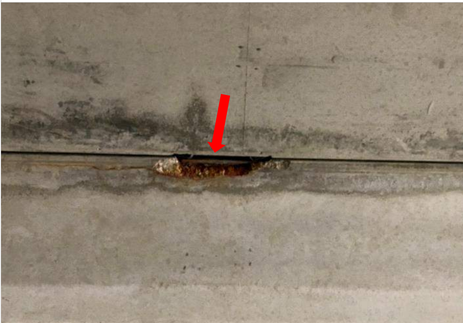
Photo 24 – Corroded double-tee shear connector noted.
