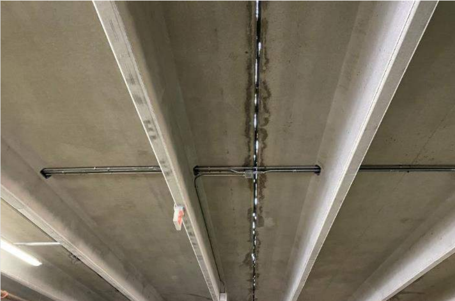
Photo 14 – Typical failed tee-to-tee joint sealant as observed from the underside at isolated locations throughout the structure. Note daylight at failed sealant.
