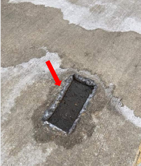
Photo 3 – Typical delaminated concrete at lifting loop pockets.
