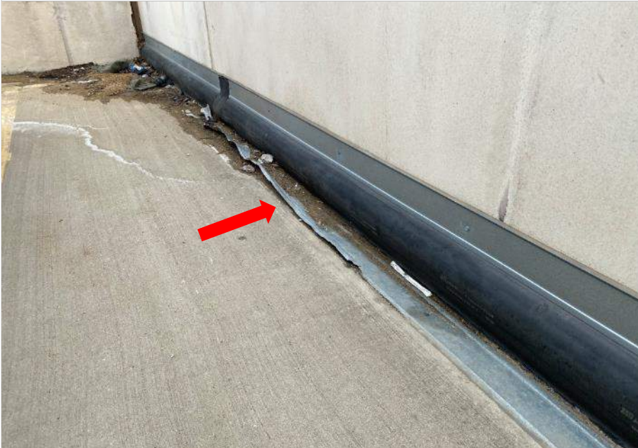
Photo 19 – Counter flashing bent and allowing water intrusion. Sealant at floor line failed.
