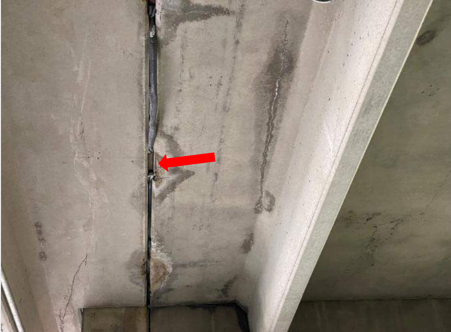
Photo 23 – Broken double-tee shear connector observed (welds broken).
