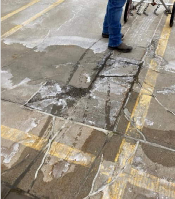
Photo 1 – Typical spalled and delaminated concrete.
