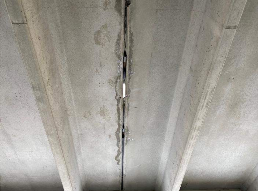
Photo 13 – Widespread failed tee-to-tee joint sealant observed.
