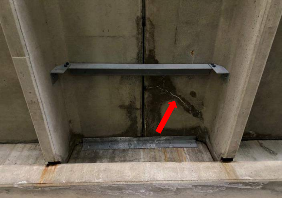
Photo 7 – Full-depth cracking and water infiltration observed at double-tee flanges that were previously repaired.
