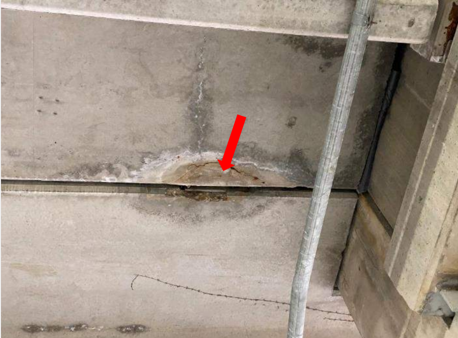
Photo 5 – Typical delaminated/spalled concrete on the underside of a tee flange.
