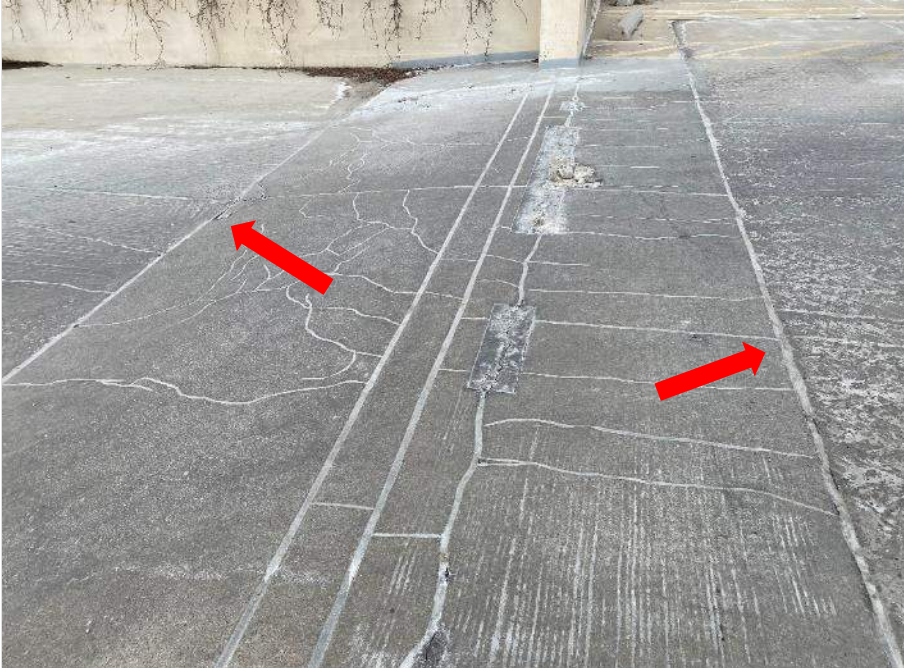
Photo 17 – Failed construction joint sealant noted throughout parking structure.
