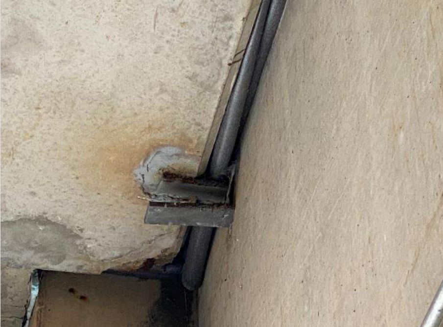
Photo 25 – Broken double-tee to wall connection observed.
