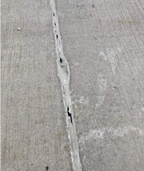
Photo 11 – Widespread failed tee-to-tee joint sealant observed.
