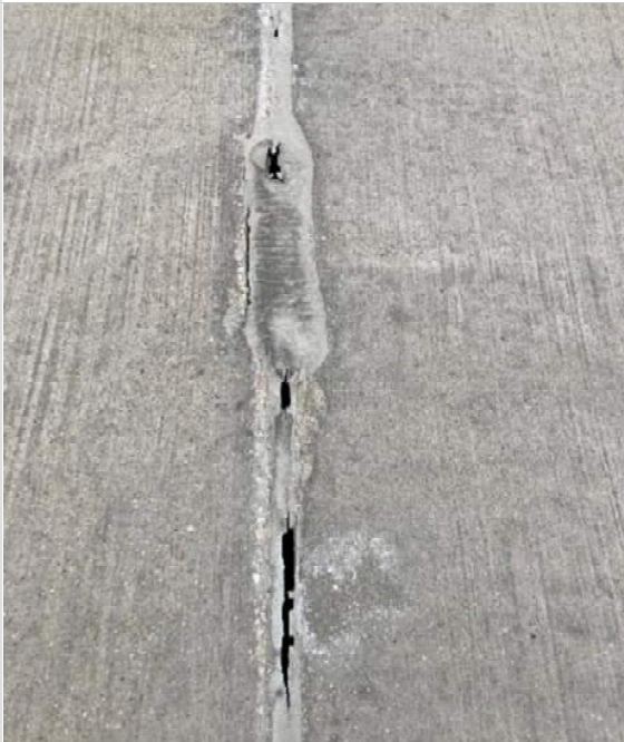
Photo 12 – Widespread failed tee-to-tee joint sealant observed.
