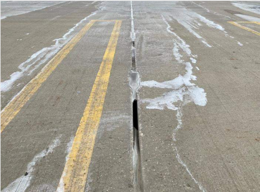
Photo 10 – Widespread failed tee-to-tee joint sealant observed.
