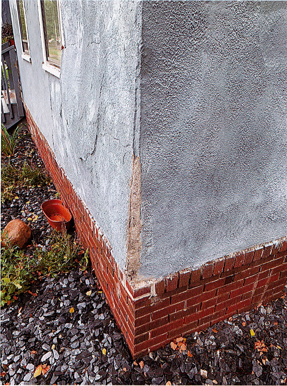
Same area as picture above except from different angle. Note how corner was patched (now damaged) but not painted.
