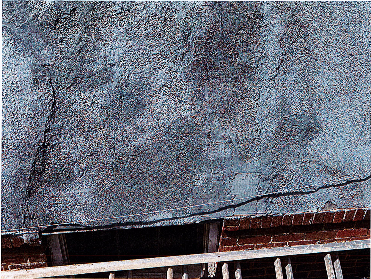
Note the exposed wood of the window well can be seen where plaster has fallen off (bottom left of picture)
