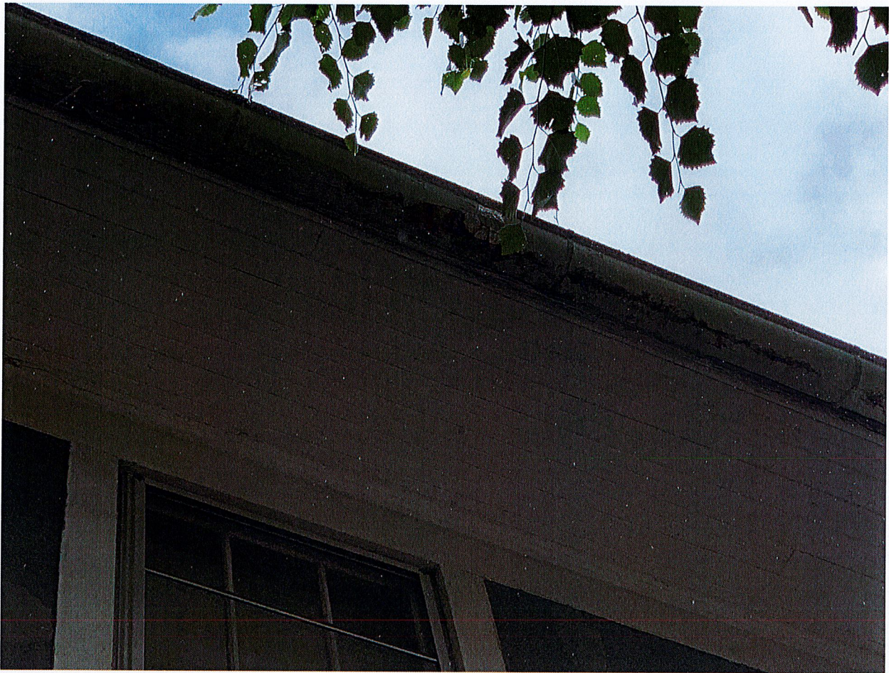
Rusted all the way through. This leakage causes flooding in my basement.
