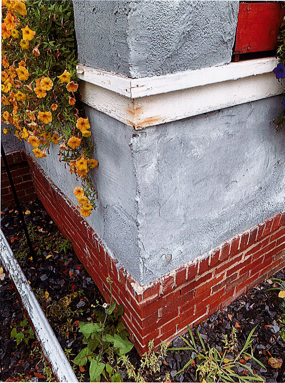
Shoddy/uneven old patchwork on front porch
