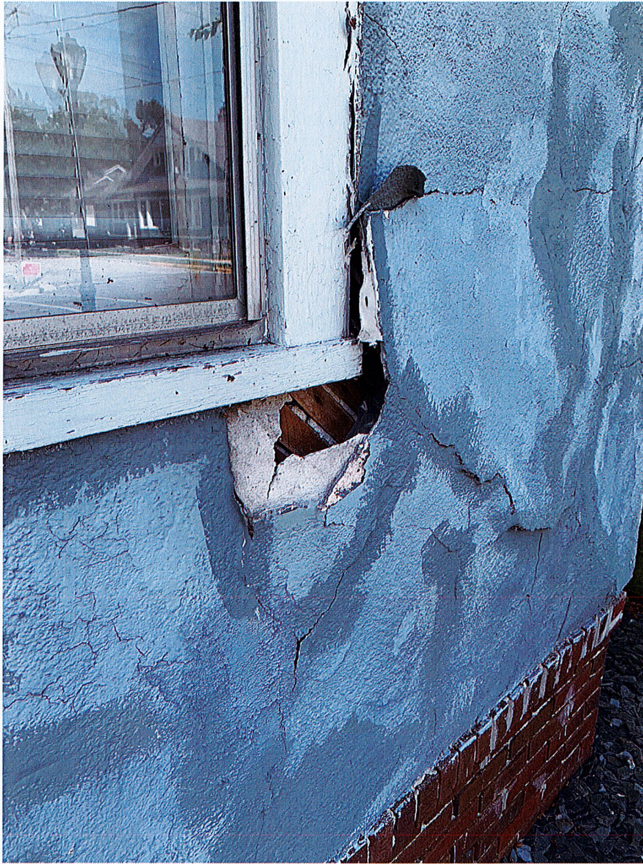
Front of house on bottom right side below window. Plaster has broken off and separated from the side of the house.
