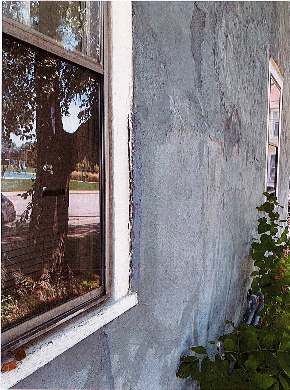
Notice the bubbling which starts about halfway up the window and goes all the way to the far window. It was caulked by the window at one point to keep water from the gutters out.
