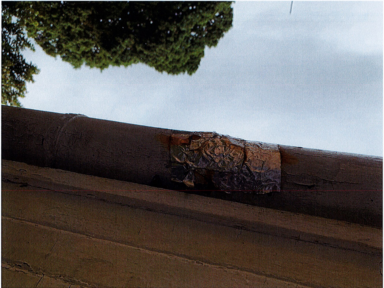
Rusted through portion of gutter over front porch that was patched with metal tape.
