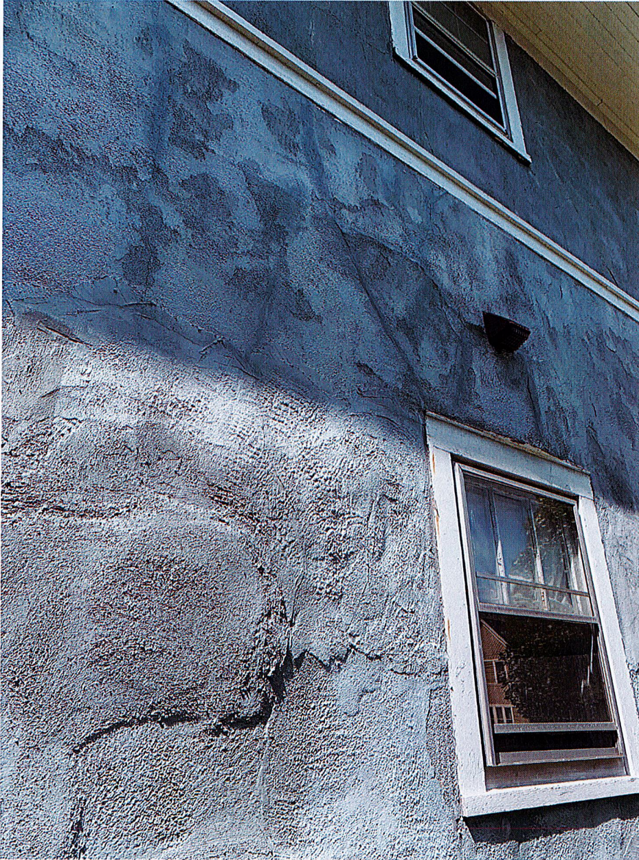
Years of patchwork, East side of home.
