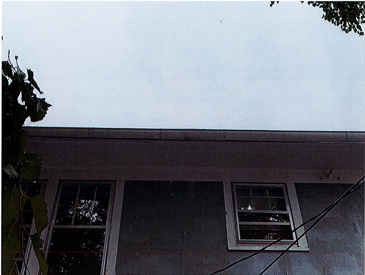
Rusted Section along West side of house. Gutters are unlevel and separated from the edge of roof. Note soffit wood work needed that is a part of the estimate.
