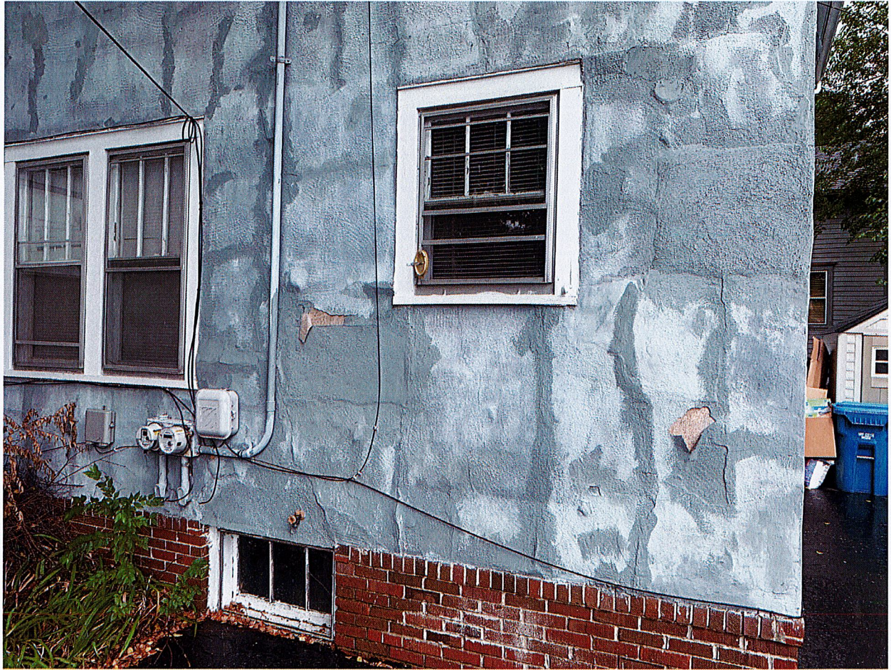
West side of house near driveway. Note the bubbling/cracking and peeling exterior.
