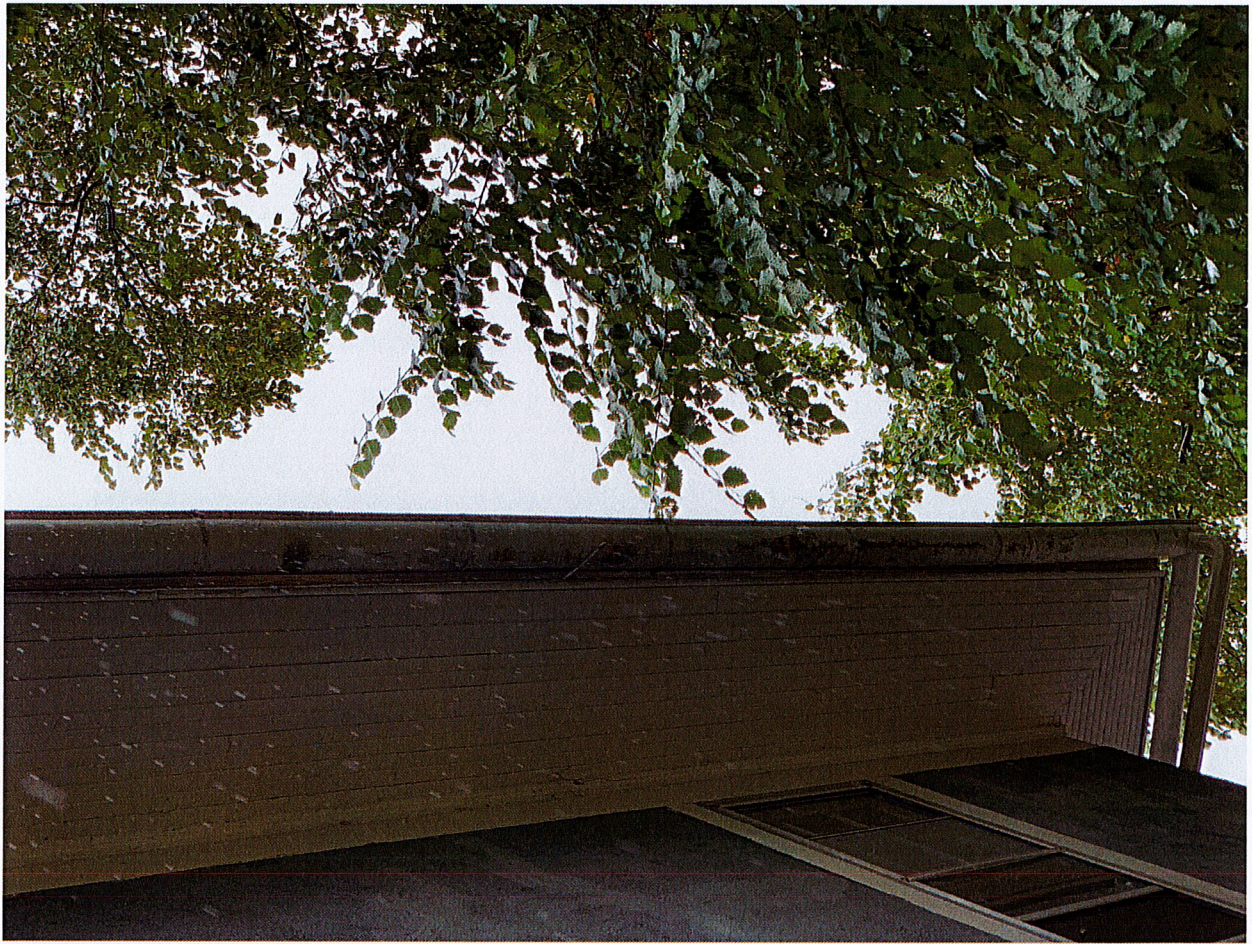
Rusted through the bottom/unlevel
