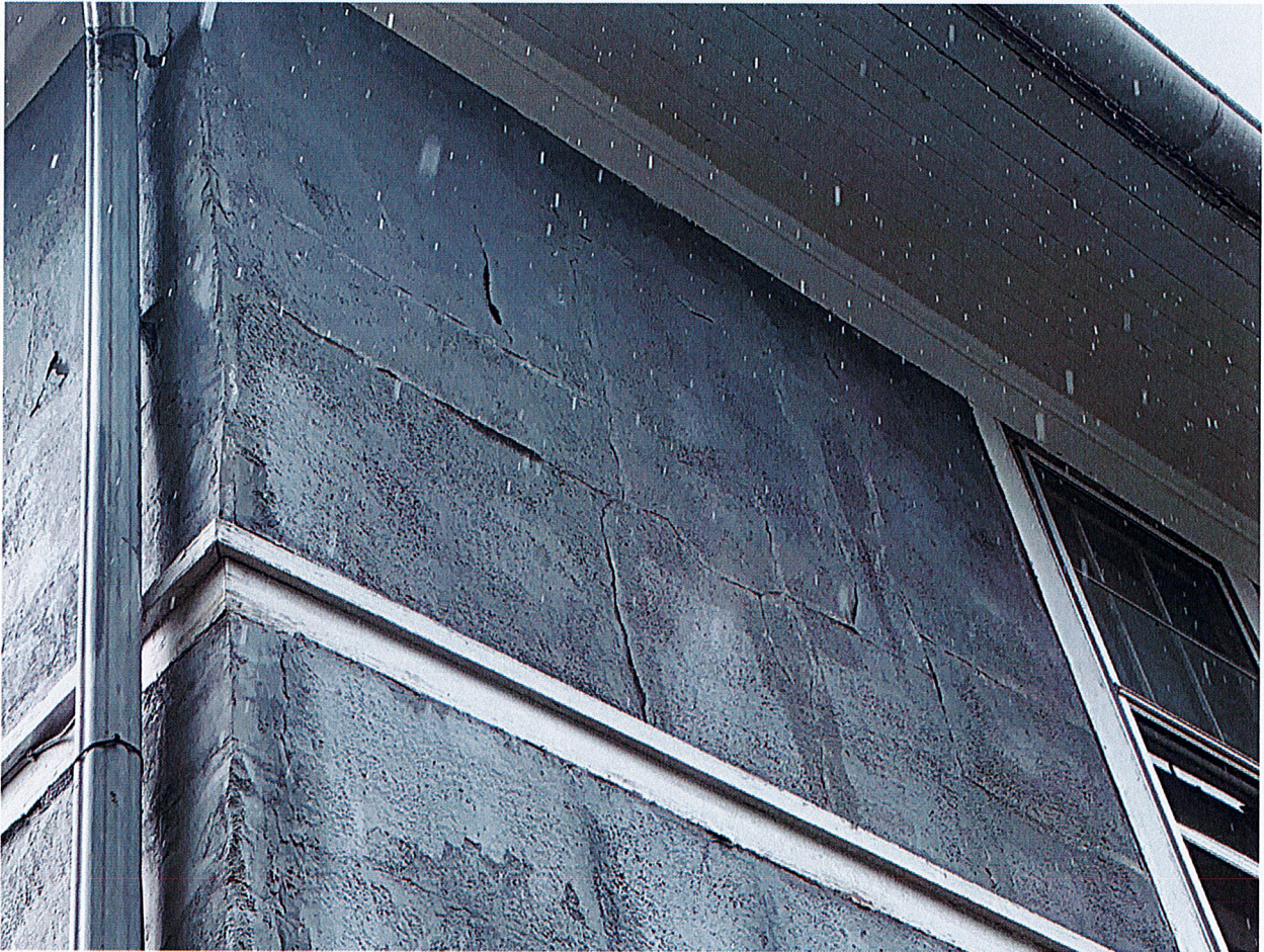
Cracks and bubbling can be found everywhere. This is on the second story near the rear SE corner of the home.
